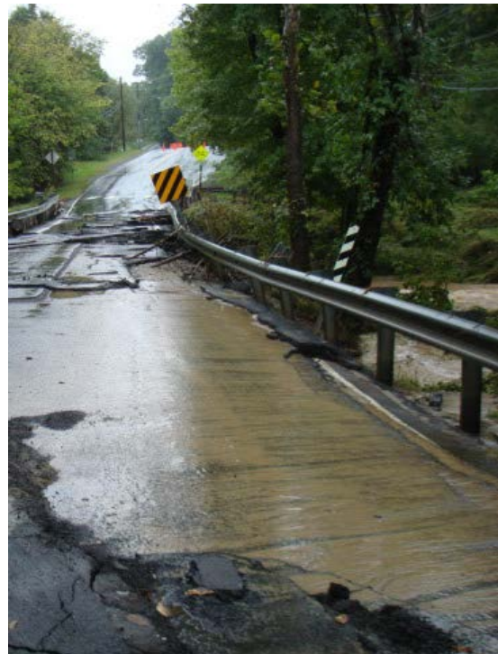
Figure 1. Damage to Hunter Mill Road in Fairfax County from Tropical Storm Lee (2011). Source: Flickr/VDOT
